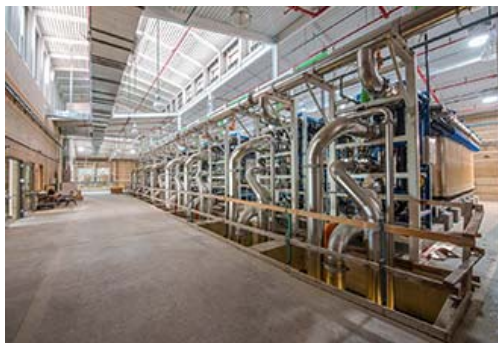
Membrane Filtration System at the Baker Water Treatment Plant
