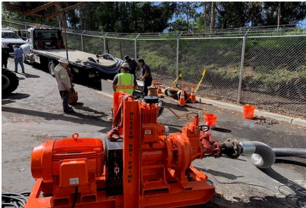
Temporary Backup Pump
