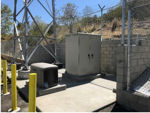
New Electrical Enclosure and Kohler Generator
