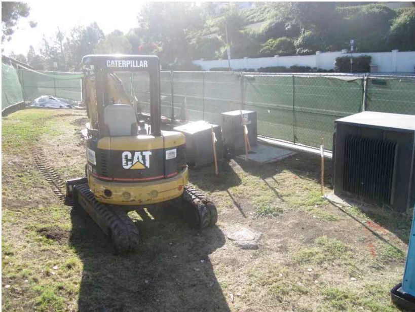
Site No. 7, Valencia Pump Station
