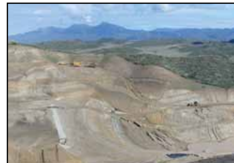
Upper Chiquita Reservoir will add 244 million gallons of local emergency water storage when completed in 2011.
